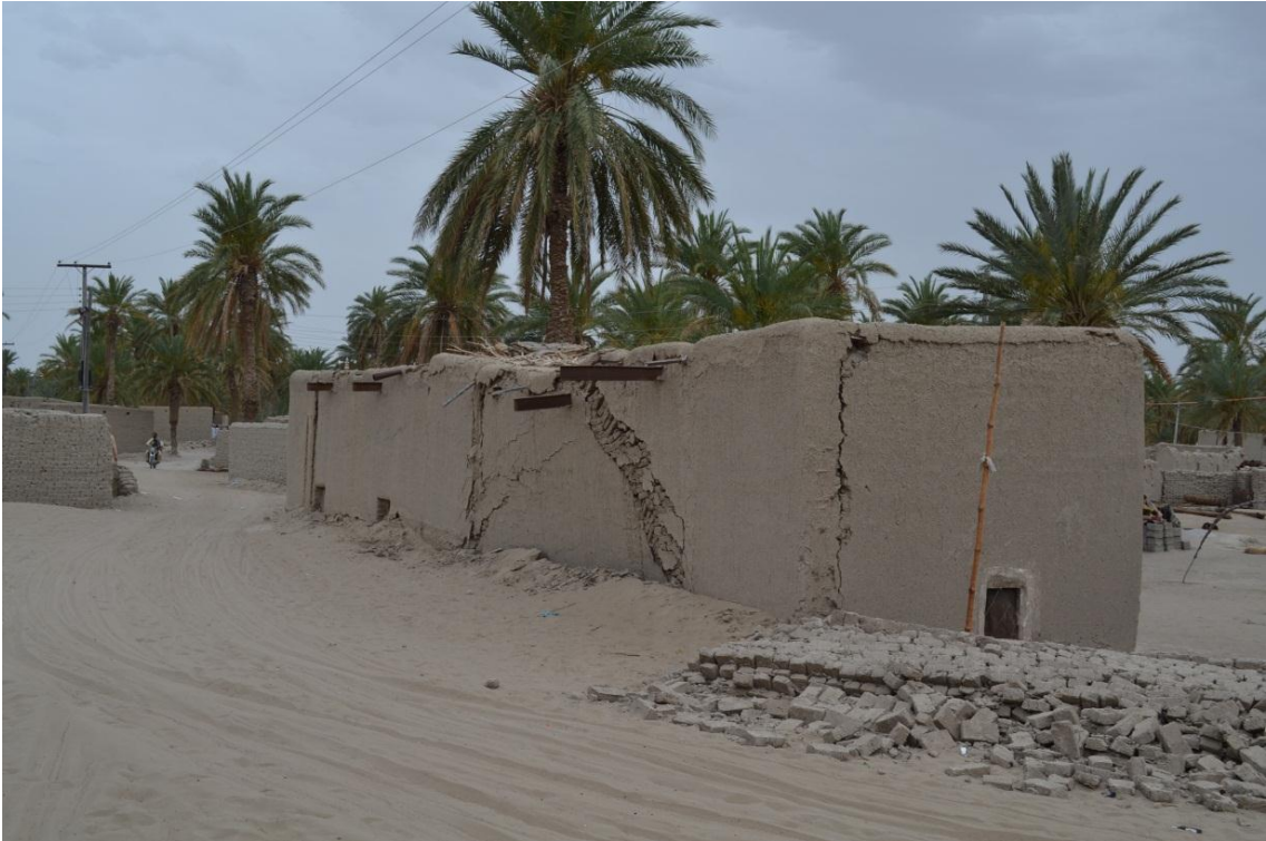
Fig. 10 Visible crack in walls in adobe buildings in Kili Kallag
