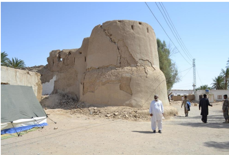
Fig. 9 View of damaged castle in FC Headquarter in Mashkel
