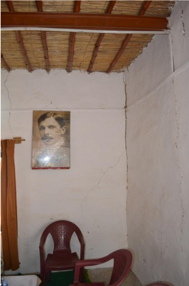
Fig. 6 Cracking in block masonry building in FC Headquarter
