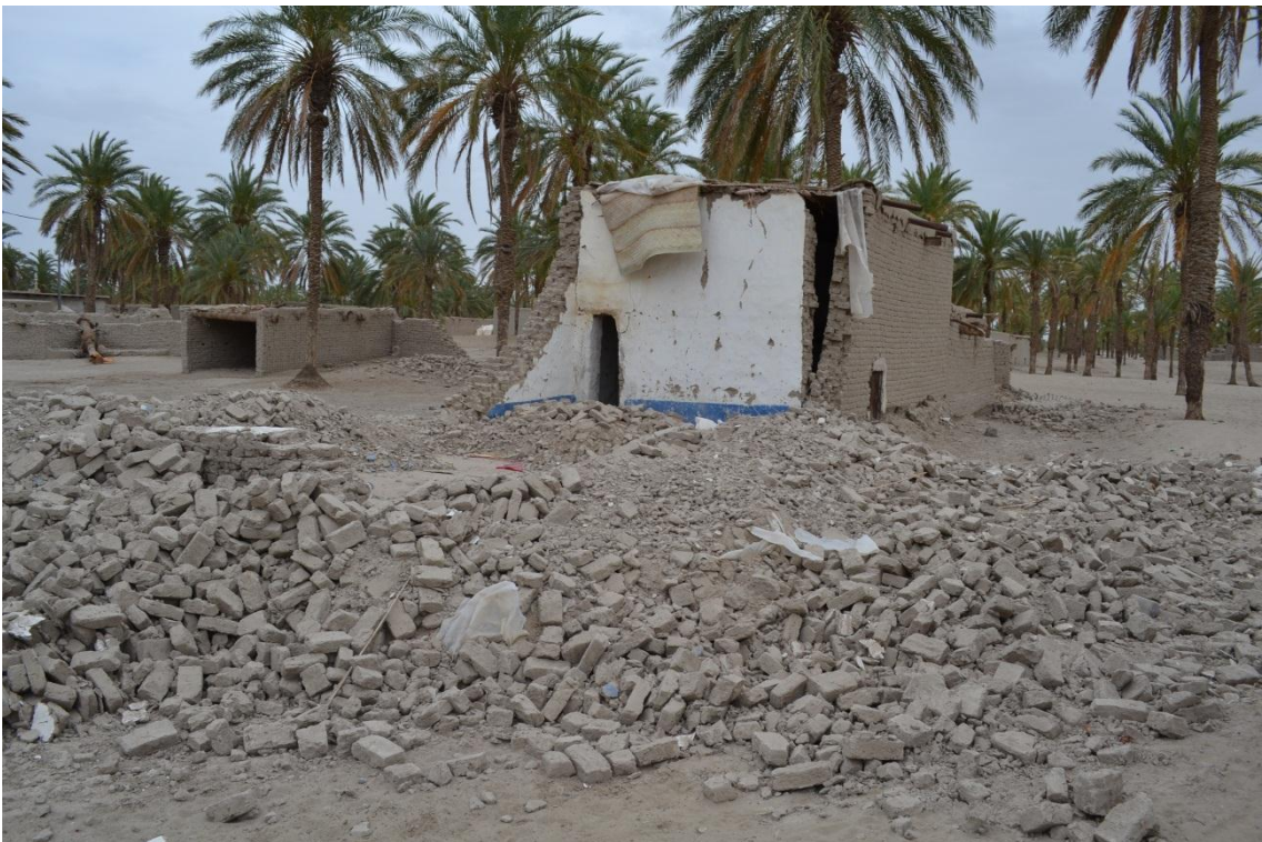
Fig. 11 Damaged adobe houses in Kili Kallag
