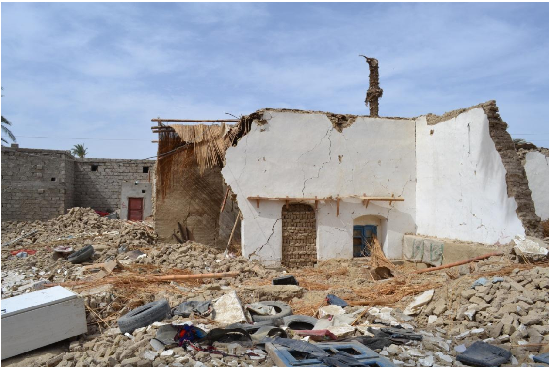
Fig. 7 Damaged adobe buildings in East Zawag
